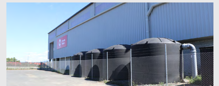
Tanks for rainwater harvesting.
